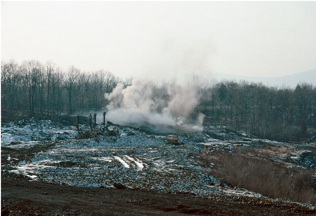
Figure 1-7 Another wartime weapon that found useful peacetime application was high explosives for blasting of rock that otherwise could not be moved.
