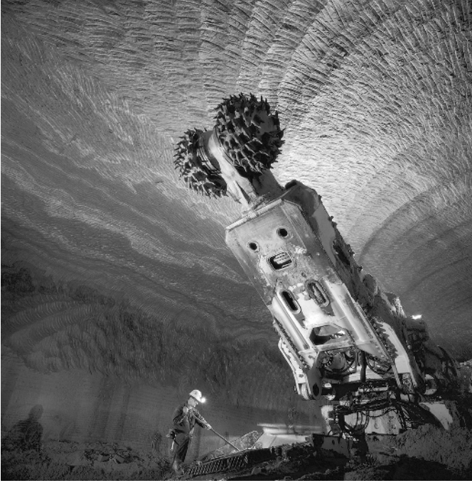
FIGURE 1-4 A mining machine with a boom-mounted cutting head. Machines such as this are use often used in potash mining to trim irregularities in the mine workings to ensure a safe working environment.
