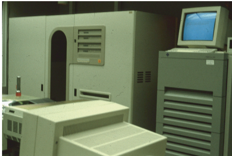
Figure 1.1q Hierarchical storage system of a PACS, consisting of a Kodak Optical Disk Library (left) with one hundred 14-inch disk platters, a RAID (right), and AMASS file management software at UCLA. Similar systems were used in later military MDIS PAC systems.
