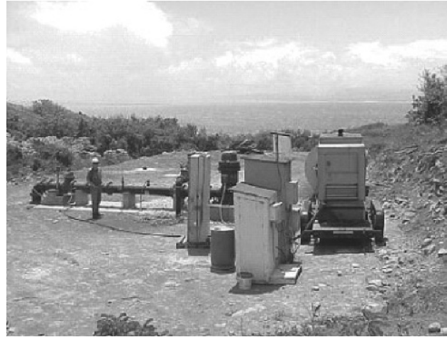
Figure 1.3 A well provides about 1.5 MGD (5.68 MLD) of water to Central Maui, HI (Courtesy of the Department of Water Supply, Maui County, HI).
