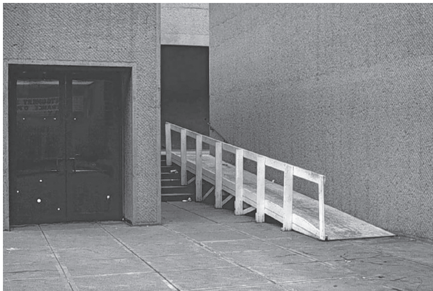
Figure 1–9: An early and unsuccessful attempt to make the Everson Museum in Syracuse, New York, accessible.
