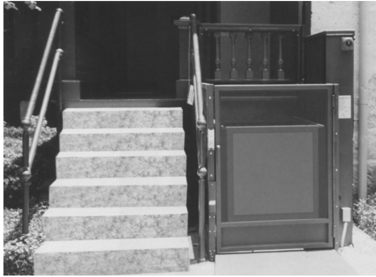
Figure 1.17. A platform-type lift installed adjacent to common stairs (Courtesy The National Wheel-O-Vator Co., Inc.).
