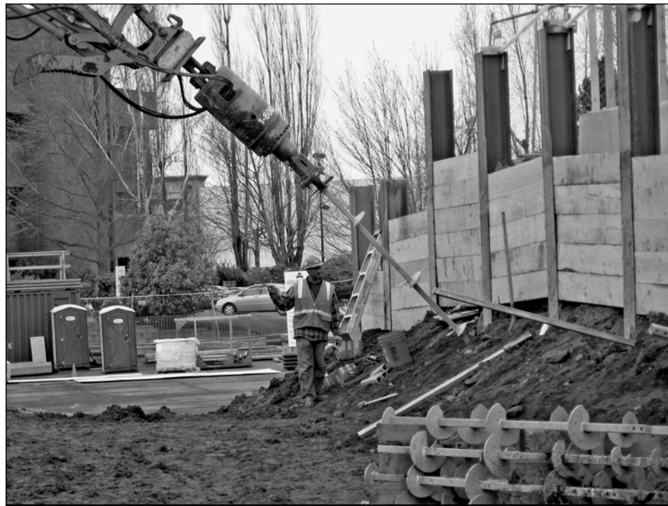
Figure 1.27 Soldier beam and lagging system with helical tie-backs (Courtesy of Earth Contact Products, Inc.)
