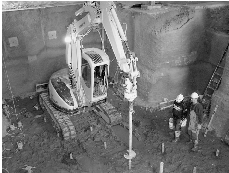
Figure 1.25 Helical pile foundation for underground MRI facility (Courtesy of Magnum Piering, Inc.)
