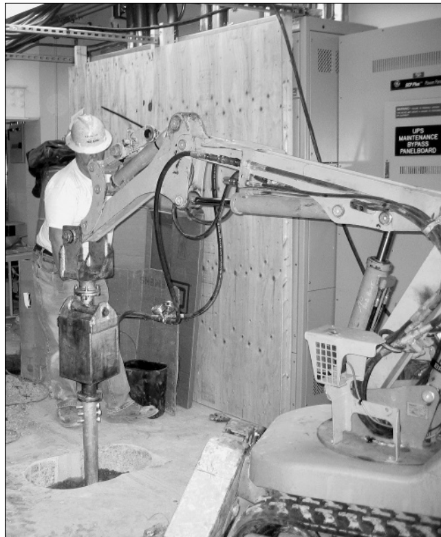
Figure 1.2 Helical pile installation in limited access area (Courtesy of Earth Contact Products, Inc.)
