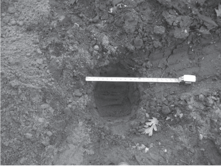
Figure 1.17 A hole is dug 12 inches in diameter by 12 inches deep, and the sides are scarified.
