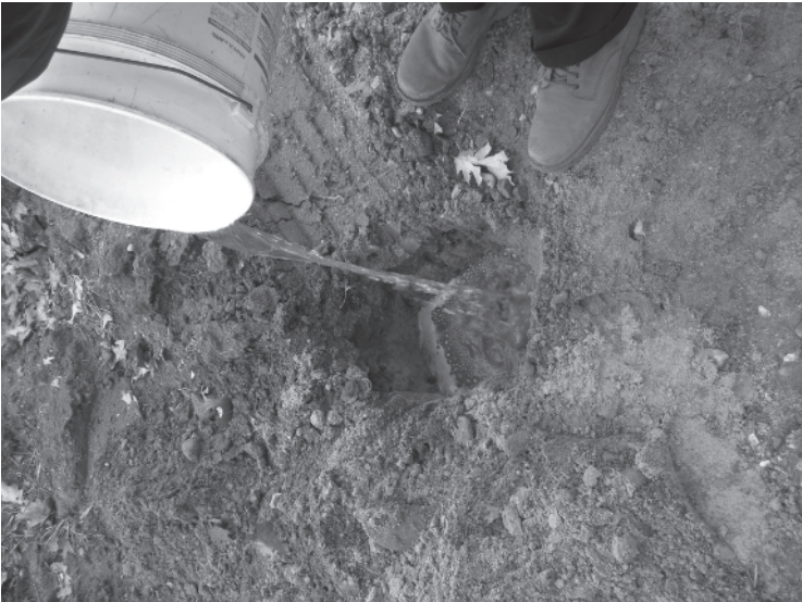
Figure 1.18 After covering the bottom of the hole with an inch or so of fine gravel, add water to the top of the hole.
