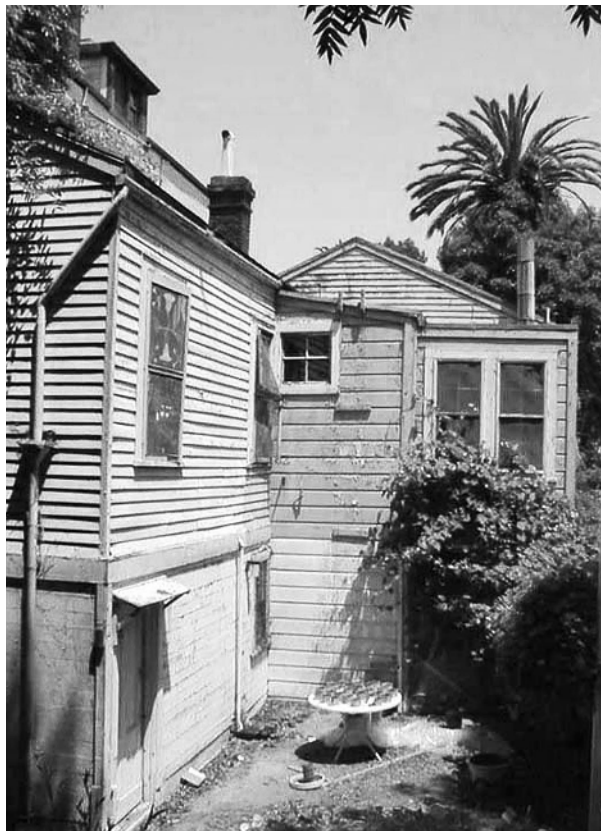
Leaking windows, lack of insulation, and obsolete systems make this building an energy hog. Source: Gelfand Partners Architects
