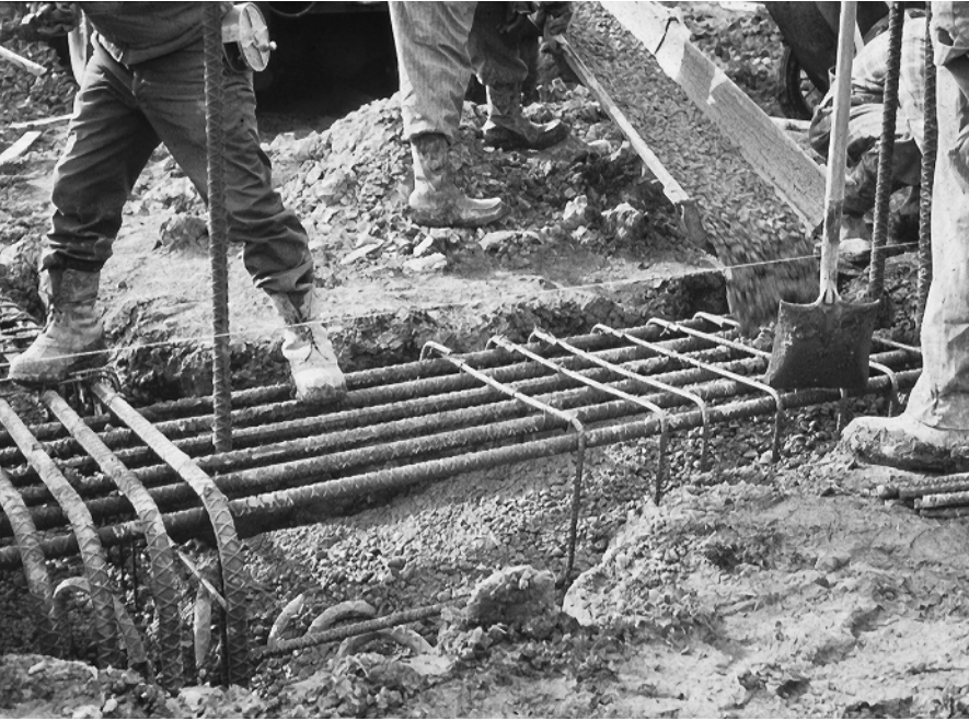
Figure 1-35 Steel and concrete have almost identical thermal rates of expansion. The steel helps the concrete resist tensile forces, and the concrete prevents the steel from rusting due to its alkaline environment. Photography by Jerry Larson.
