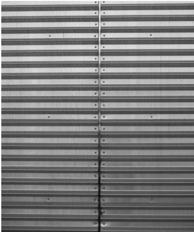
Figure 1-49 Hot-dipped galvanized steel panels at the State Street Village graduate residence hall, Illinois Institute of Technology, Chicago, Illinois. Building designed by Helmut Jahn (2003). Photography by Jim Postell.
