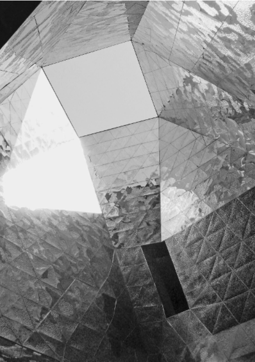
Figure 1-2 The faceted soffit is clad in polished stainless steel with a pockmarked texture. Barcelona Forum, Barcelona, Spain, designed by Herzog & de Meuron (2004). Photography by Audrey de Filippis.
