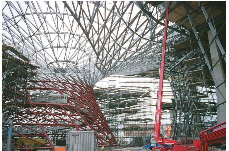
Complex roof structure of the BMW Welt building in Munich by Coop Himmelb(l)au architects and Bollinger + Grohmann structural engineers. See 'Form, Force, Performance: Multi-Parametric Structural Design' on page 20.
