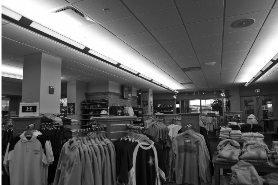
Figure 1-14a Mounting indirect luminaires close to the ceiling can reduce overall system efficacy.
