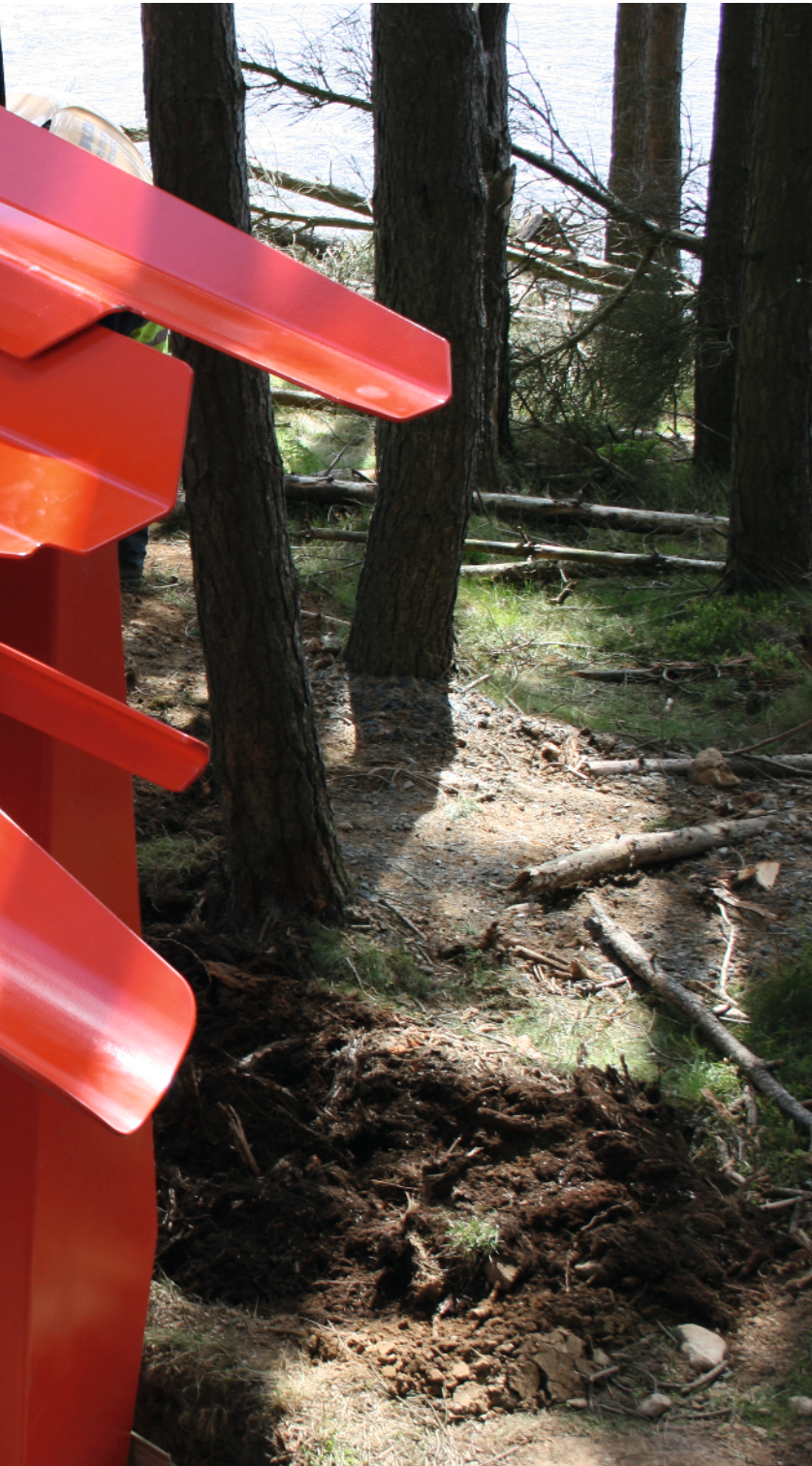
The assembled construct. 55/02 installed on site at Cock Stoor, Kielder Water, and seen from above. The image shows a detail of the assembly of painted roof components. Photograph: Bob Sheil. © sixteen*(makers).
