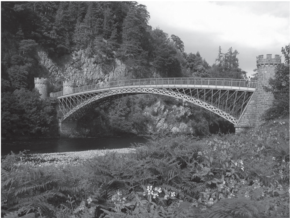
Figure 1.21 Craigellachie Bridge, 45 m span, over the Spey River, Scotland, 1815 (Source: Photograph by Craig Williams/ https://commons.wikimedia.org ).
