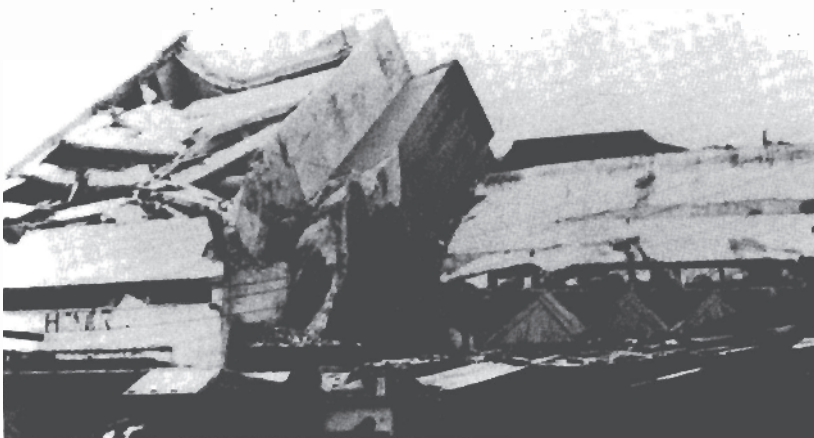
Fig. 1.4 Failure of structural wall resulting from inadequate flexural and shear strength (1990 Philippine earthquake). (Courtesy of EQE Engineering Inc.)
