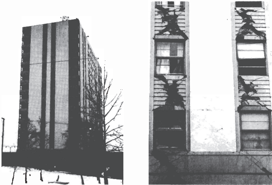
Fig. 1.5 Failure of coupling beams between shear walls (1964 Alaskan earthquake). (Courtesy of the American Iron and Steel Institute.)
