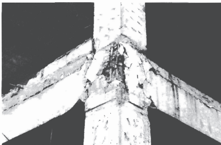
Fig. 1.7 Beam-column connection failure (1990 Philippine earthquake). (Courtesy of T. Minami.)
