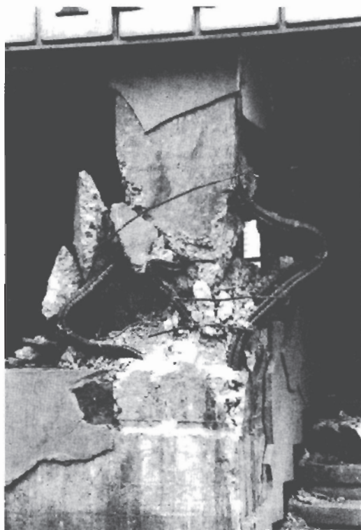
Fig. 1.2 Confinement failure of column base of 10-story building. (Courtesy of EQE Engineering, Inc.)
