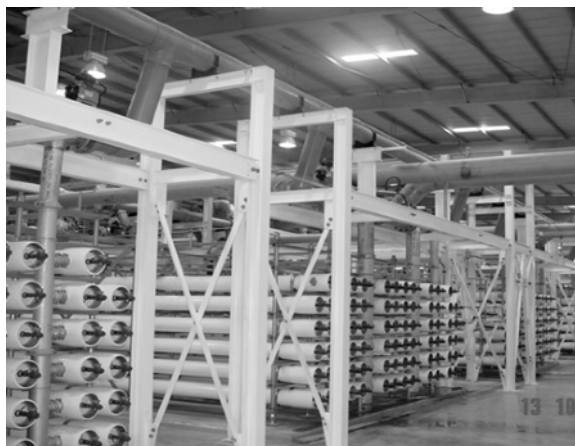
Figure 1.12 RO portion of wastewater reclamation and reuse plant in Kuwait.
