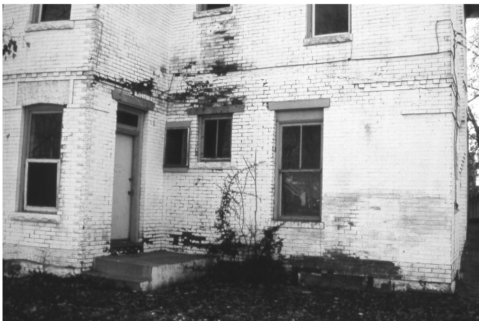
Figure 1-3 Various visual and physical clues indicate several changes in this entranceway: a porch roof and decking have been removed; windows have been added or modified; and drainage/moisture problems have occurred. These clues are given by changes in the brick, window sills, and lintel construction materials, as well as missing or peeling paint.
