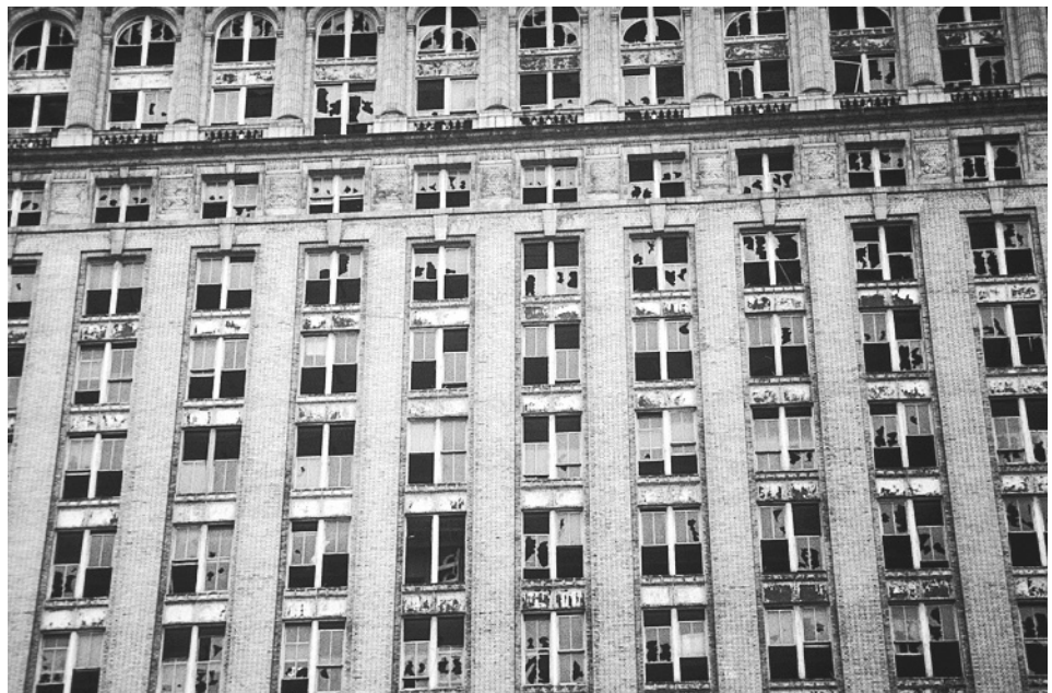
Figure 1-2 Unsecured and vacant buildings invite vandalism and unwanted trespassers, as the damage to this building demonstrates.
