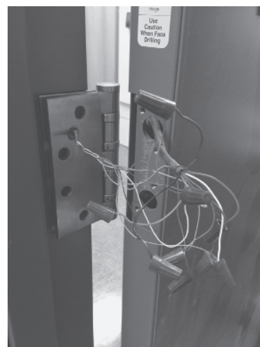
FIGURE 1.36 Electric Transfer Wired to Door
