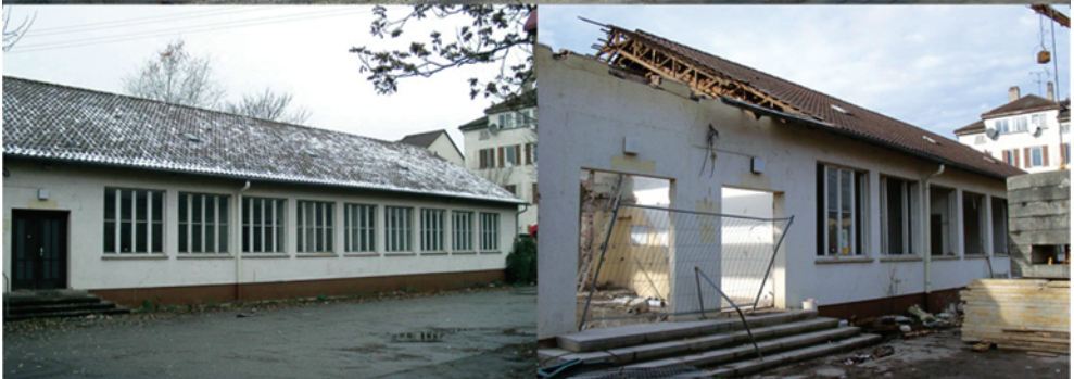
Figure 1.2 The ebök passive standard office building in Tübingen, Germany after (top), before (bottom left) and during (bottom right) renovation work (Photo: eboek GmbH, Tuebingen).
