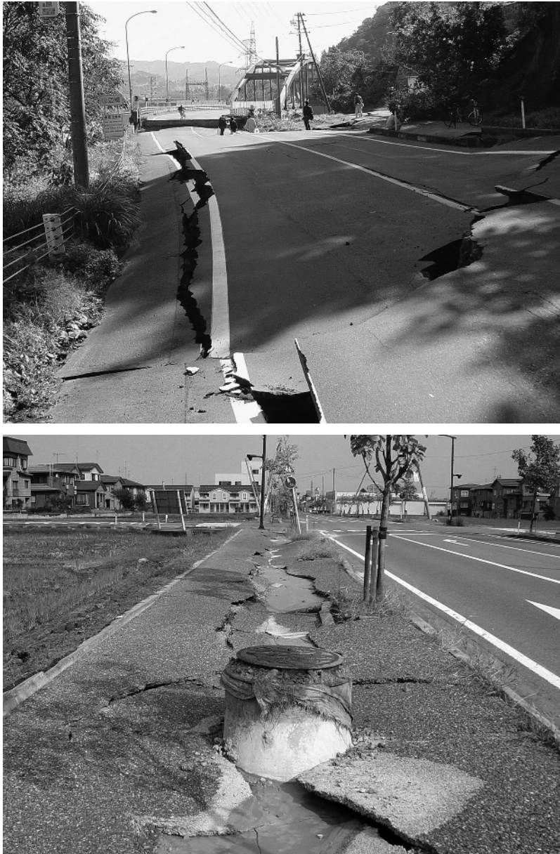
Figure 1.3 Road damage following a 6.8 magnitude earthquake in Chūetsu on October 23, 2004, which occurred in Niigata Prefecture, Japan. The road and other routes suffered heavy damage due to landslides and faulting that resulted from liquefaction. (Source: Tubbi [CC-BY-3.0-br ( http://creativecommons.org/licenses/by-sa/3.0/deed.en )], via Wikimedia Commons; http://commons.wikimedia.org/wiki/File:Chuetsu_earthquake-Yamabe_Bridge.jpg )
