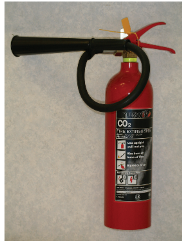
Figure 1.5 A fire extinguisher.
