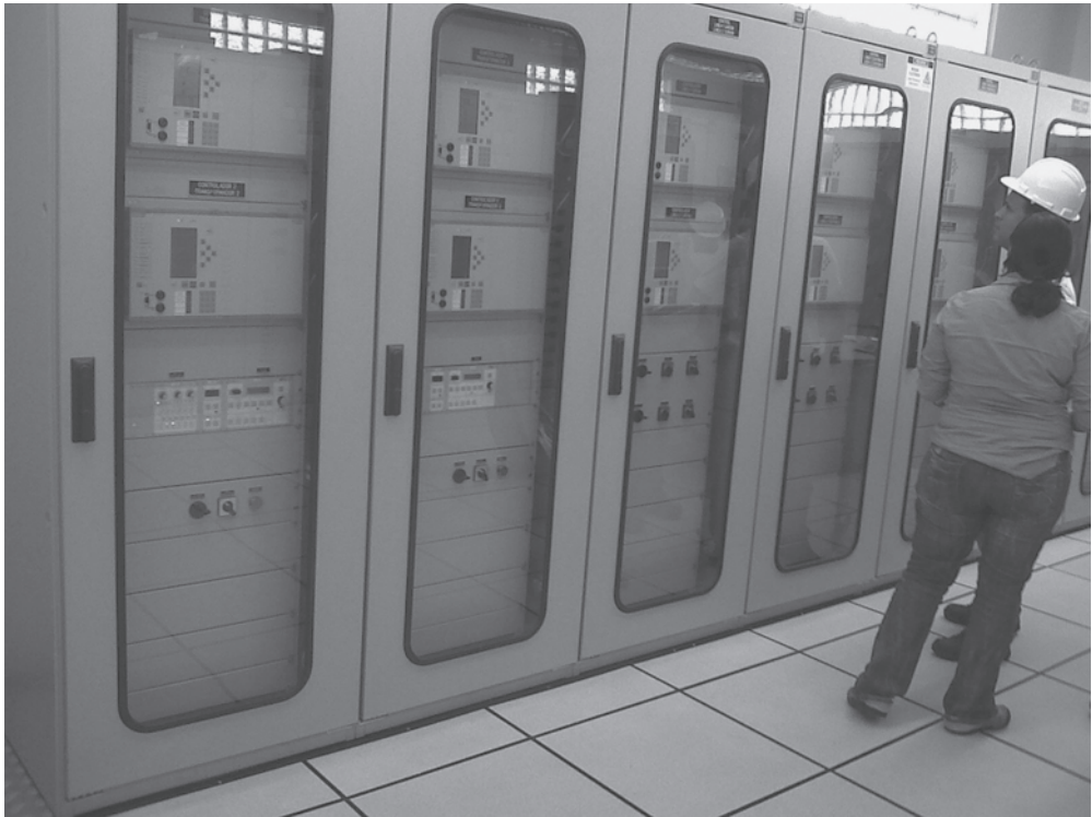
Figure 1.6 Control cubicles of a modern SAS. Source: © Corpoelec. Reproduced with permission of Corpoelec
