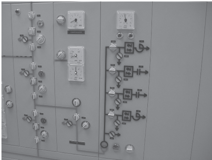
Figure 1.3 Substation primary arrangement shown outside control cubicles. Source: © Corpolec. Reproduced with permission of Corpolec
