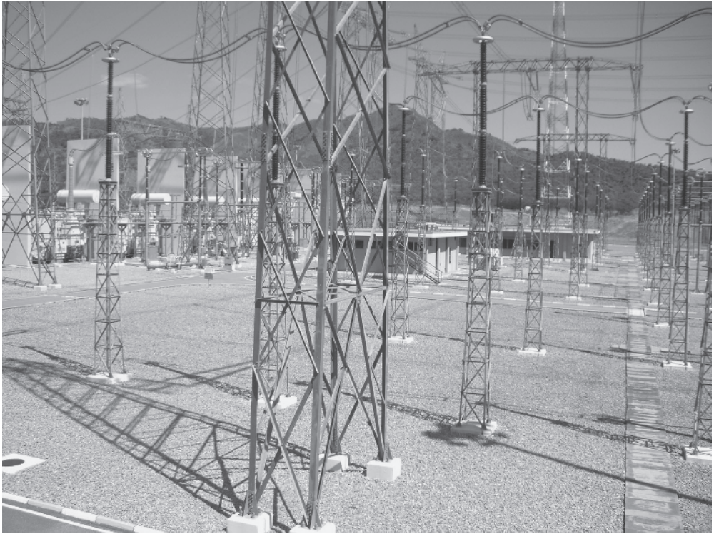
Figure 1.1 View of a 765 kV electric substation. Source: © Corpoelec. Reproduced with permission of Corpoelec
