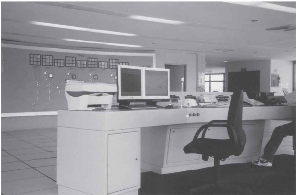
Figure 1.7 Operation desk of a modern SAS. Source: © Corpoelec. Reproduced with permission of Corpoelec
