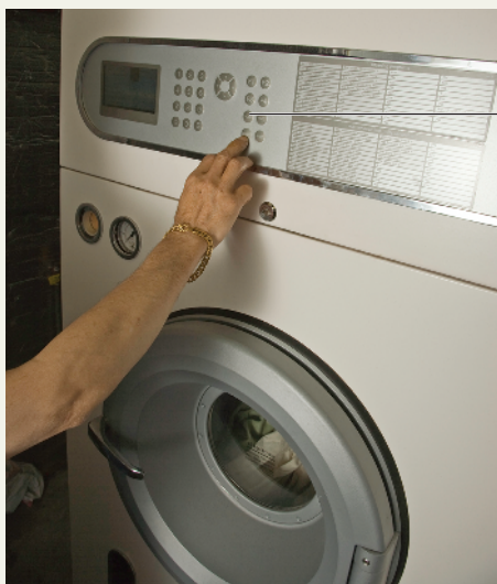
Controls for regulating flow of dry-cleaning liquids
