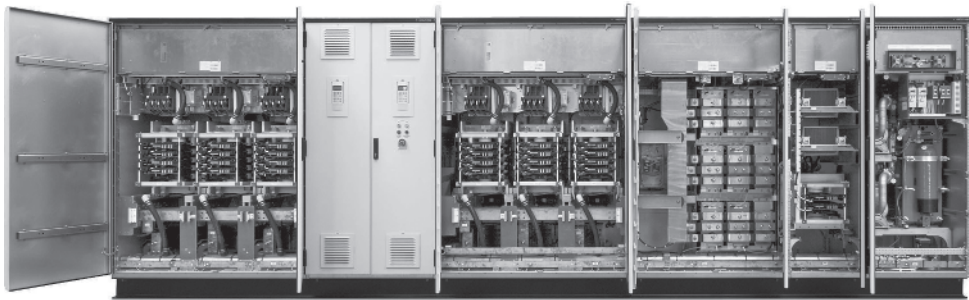
(a) ACS6000 with an active front end, the terminal and control unit, the inverter unit, the dc-link capacitor bank, a voltage limiter and the water cooling unit
