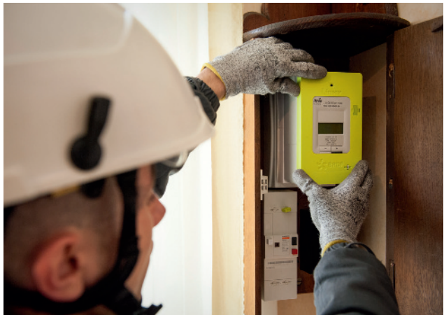
Installation of a smart electricity meter in France, 2011 Linky, the meter promoted by EDF, France's foremost electricity supply company, is intended as a first step towards a better management of the electricity grid.
