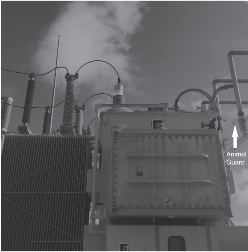
Figure 1.17 Animal guard around the top of the transformer low voltage bushing.
