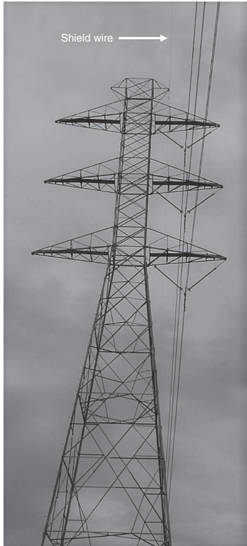
Figure 1.13 Shield wire on a single-circuit 345 kV transmission line. (Photo: Courtesy of Mr. Genardo Corpuz, Lower Colorado River Authority, USA.)
