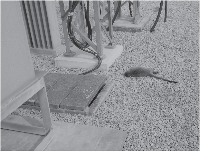
Figure 1.14 A monkey that made contact with energized equipment in a substation and created a fault. (Photo: Courtesy of Mr. Emmanuel Raubenheimer, Eskom, South Africa.)
