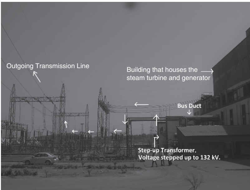
Figure 1.21 Generator step-up transformer is transforming the low voltage output from the steam turbine generator to 132 kV and interconnecting the power station to the transmission network. (Photo: Courtesy of Mr. Dip Kumar Das, Development Consultants Private Limited, India.)
