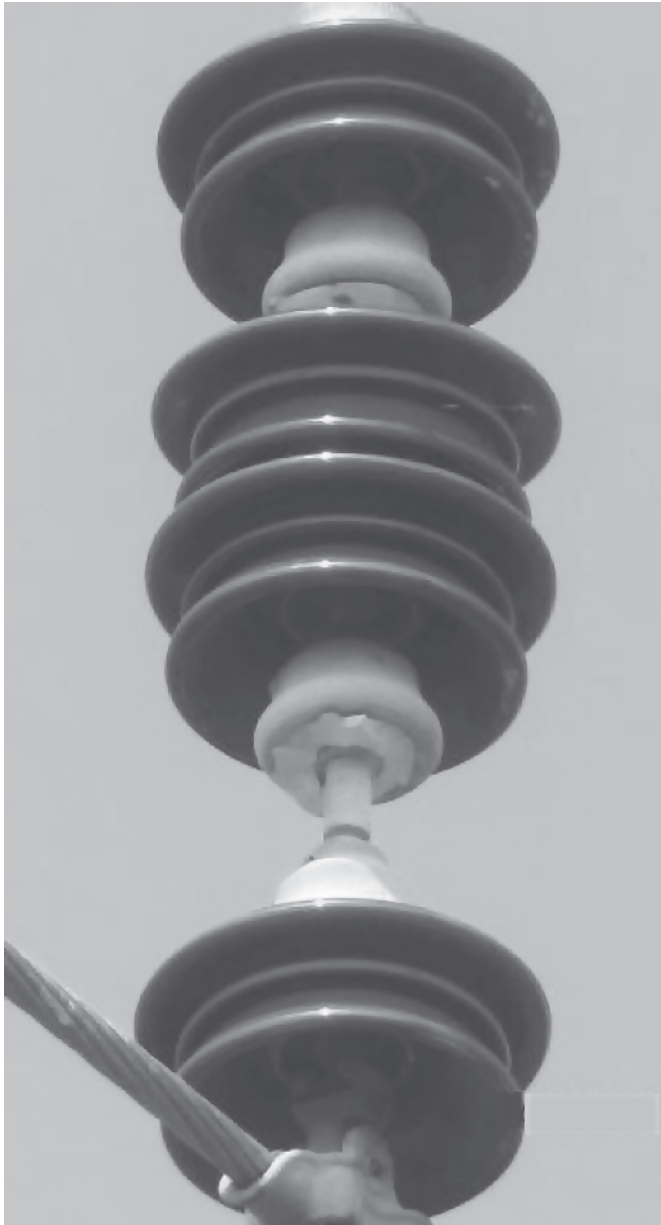
Figure 1.9 Overvoltage due to lightning strike on a 69 kV transmission line resulted in a flashover and a phase-to-ground fault. The insulator string was found to be damaged with multiple ceramic disks missing. (Photo: Courtesy of Mr. Genardo Corpuz, Lower Colorado River Authority, USA.)
