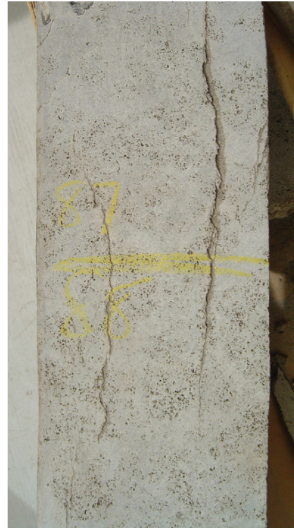
Figure A1d1.2 Two rough, parallel, high-angle extension fractures in a vuggy limestone, striking oblique to the slab surface (angling into the plane of the photo towards the left). The oblique strike exaggerates the fracture width and irregularity. Fracture dimensions on a slab plane are apparent dimensions unless the fracture strikes normal to the slab surface. Top and bottom fracture terminations are blind within a homogeneous lithology. Slab from a four-inch diameter core; uphole is towards the top of the photo.
