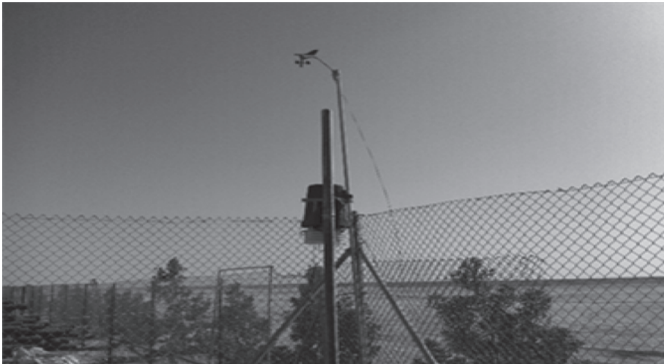
Figure 1.5 Weather station close to the SFCW cells. [5]
