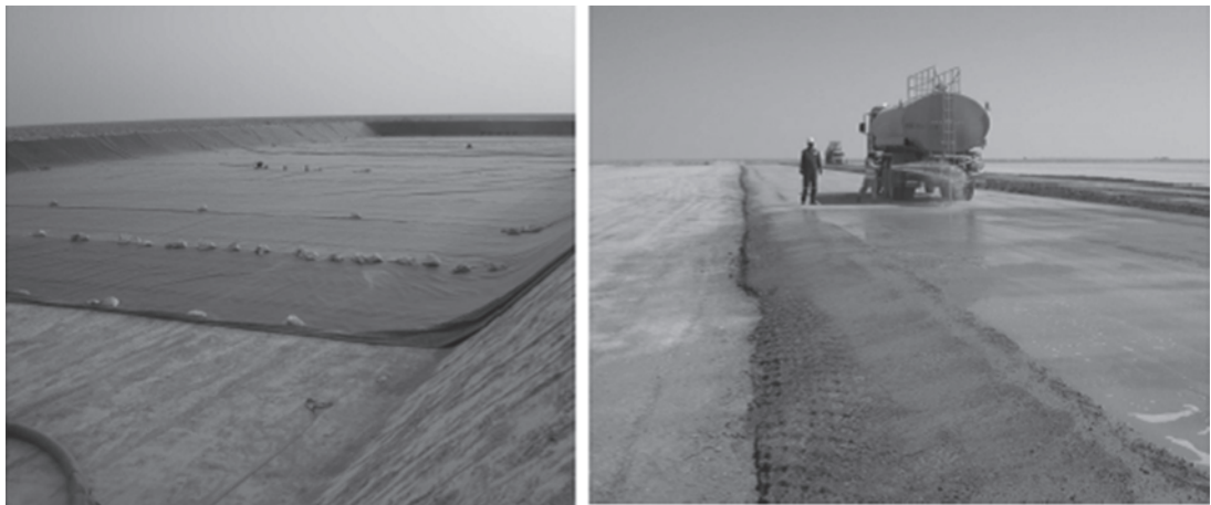
Figure 1.3 Installation of the HDPE liner in the buffer pond (left) and of the mineral sealing layer in the wetland cells (right).
