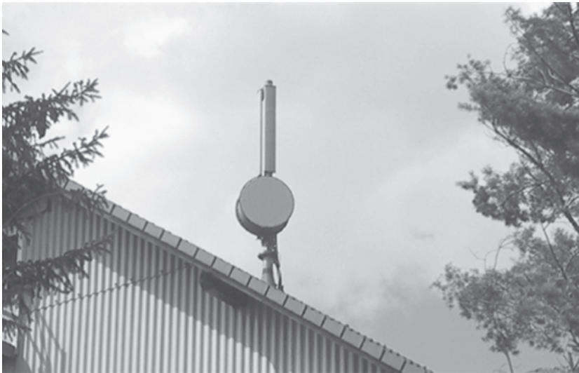
Figure 1.19 A typical antenna of a GSM base station. The optional microwave directional antenna (round antenna at the bottom of the mast) connects the base station with the GSM network. Source: Martin Sauter. Reproduced by permission of Martin Sauter.
