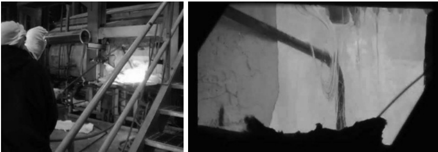
Figure 18. Left: First Water Lance Readied after GLB Superstructure Removed; Right: inserted (R)
