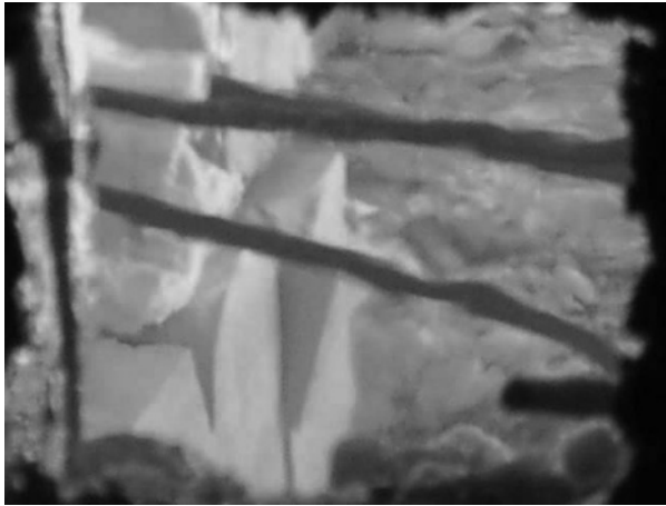
Figure 23. Interior View as Work Nearing Completion. Note: Due to the rapid exposure of the large tank wall block into the operating furnace high temperature environment, some block corner spalls occurred.
