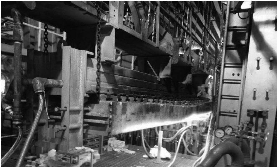
Figure 12. Old B Arch Removal from the Waist, with New B Arch being Set in Place from the Right Side
