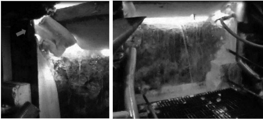
Figure 21. Left: Area of Concern in the GLB Furnace Inside Corner; Right: During Demolition. Bright orange spots of hot glass can still be seen on the right side.
