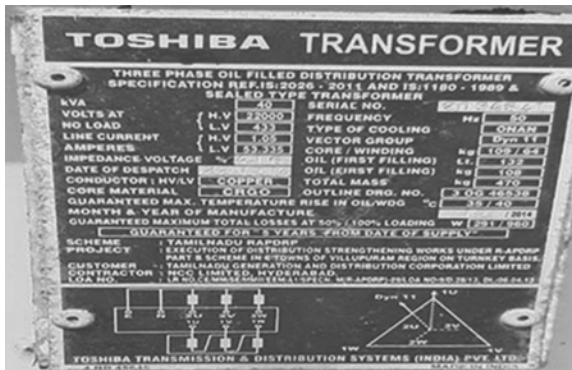
Figure 1.23 Name plate details of transformer (Courtesy: Toshiba).
