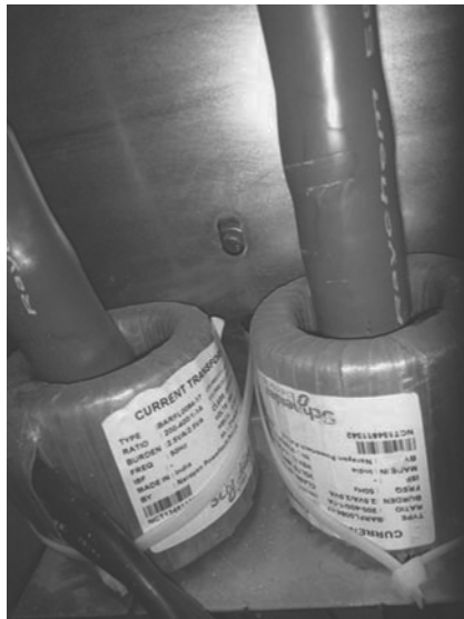
Figure 1.76 CTs at 11 kV (Courtesy: Schneider Electric).
