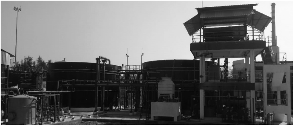
Figure 1.9 An MBBR plant.
