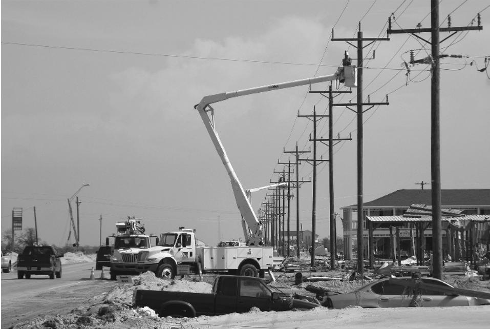
Figure 1-9 The damage of electricity infrastructure (an agent-generated demand) in Crystal Beach, TX, after Hurricane Ike created the need to replace power poles (a response-generated demand). Greg Henshall/FEMA. http://www.fema.gov/media-library/assets/images/54764
