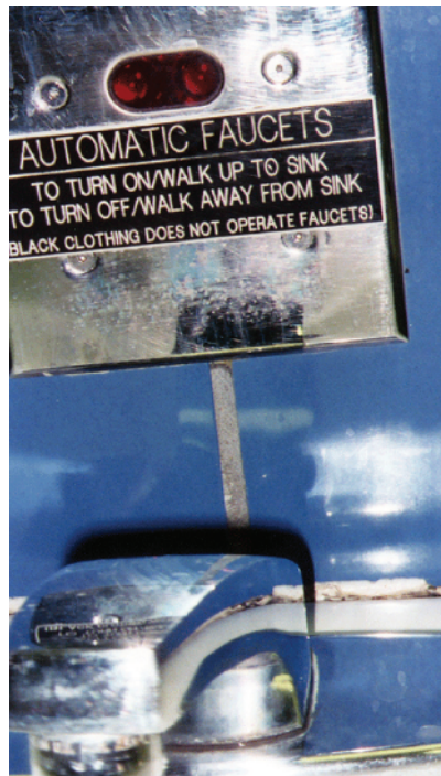
Figure 1.10 A sign in the restrooms at the Cincinnati airport
