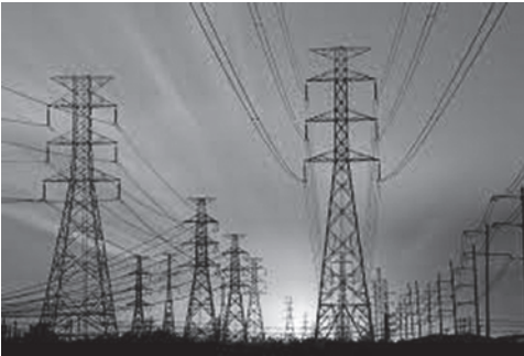
Figure 1.11 The electric power grid consists of an interconnected network of power generation stations, transmission lines, substations, and power distribution stations. China is currently the largest producer of electric energy followed by the United States.
