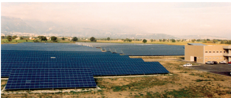
Figure 1.14 The grid-connected system (3.3 MWp) in Serre, Italy. The installation was commissioned in 1995 (Photo: ENEL)
