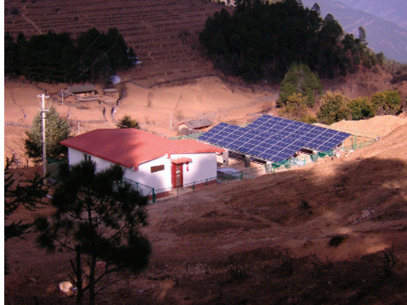
Figure 1.7 A 6 kWp stand-alone AC installation with a battery in the Chinese village of Doncun-Wushe (Photo: Shell Solar/SolarWorld)
