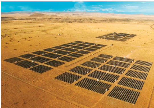
Figure 1.16 The grid-connected system in Springerville, Arizona. Currently 4.6 MWp, the capacity of this installation is being expanded incrementally to around 8 MWp (Photo: Tucson Electric Power Company; www.greenwatts.com )
