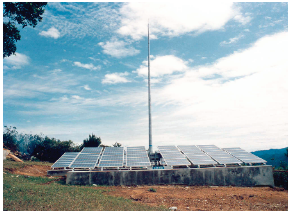
Figure 1.8 PV telecommunication installation at a remote location in Sipirok, Indonesia (Photo: Siemens)
