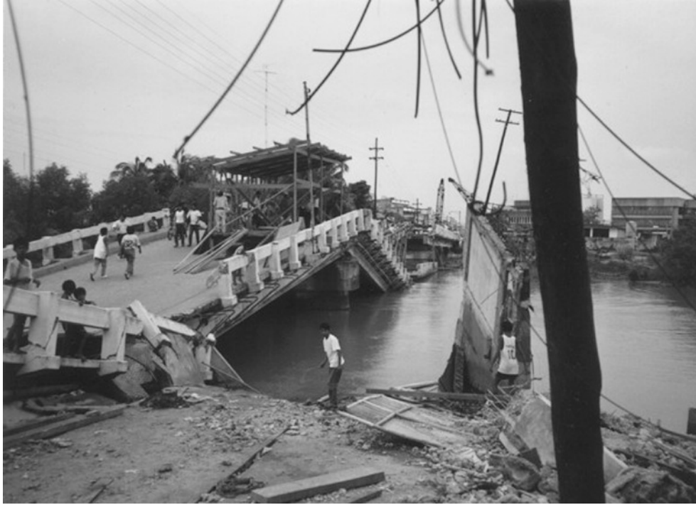
Figure 1.5 A bridge located in Dagupan, Philippines, that was damaged by an earthquake in 1990.
