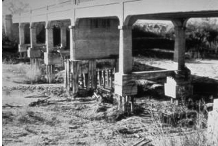
Figure 1.4 Scour of bridge piers caused by increased flow rates that erode the supporting soil resulting in changes to the bridge's boundary conditions (source: US Geological Survey).
