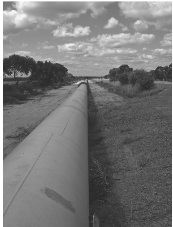
Figure 1.8 A Pipeline in the Goldfields Water Supply Scheme, Perth, Australia (Source: http://en.wikipedia.org/wiki/Image:Goldfields_Pipeline_SMC.JPG )
