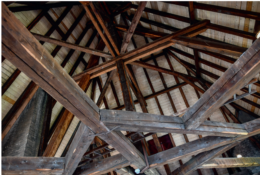
Figure 1.7 A roof structure detail from a 13 th century German castle showing original and refurbished timbers and plank covering.
