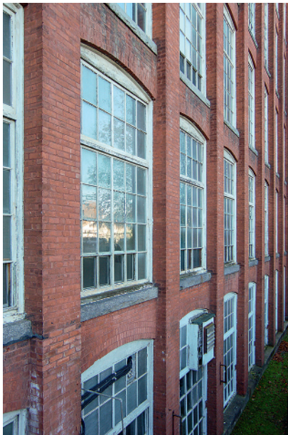
Figure 1.14 Exterior walls of an industrial mill building in Easthampton, Massachusetts, showing the common brick exterior wall and its large window openings.
