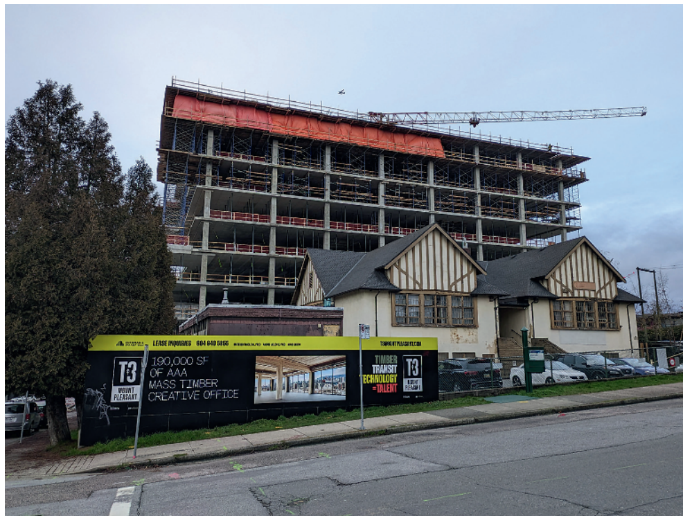
Figure 1.27 A 190,000 ft 2 mass timber building is announced for construction on a billboard right next to a concrete frame that rises in the adjacent lot in Vancouver, BC.
