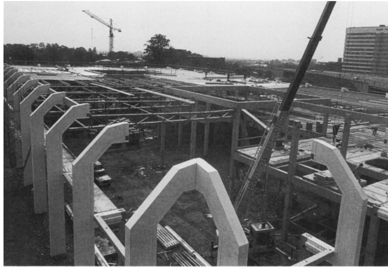
Figure 1.25 Profiled white concrete columns supporting a steel roof (courtesy of Crendon Structures Ltd).
