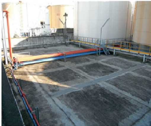
Figure 1.3. Retention basin of an oil storage tank
