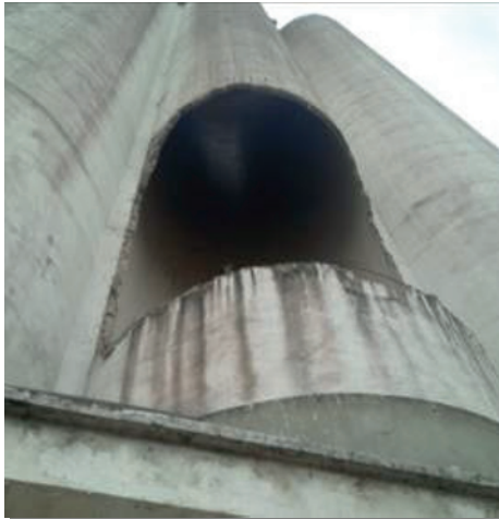
Figure 1.12. Opening of the skirt of the silo following the implementation of an internal lining
