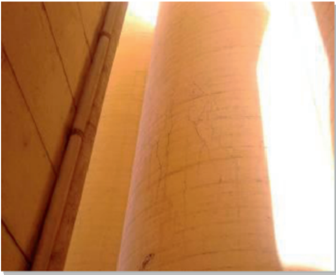
Figure 1.13. Vertical cracking of the skirt of the cylindrical silo
