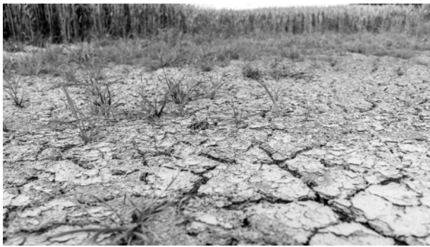
Figure 1.2. Worsening of soil condition (France)
