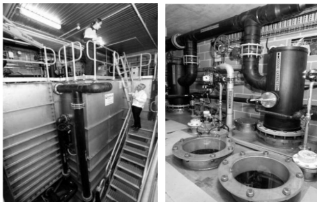
Figure 1.25. Reuse station equipment
