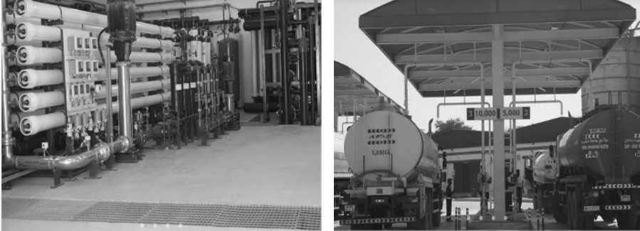
Figure 1.12. Reverse osmosis membrane and service station for reused wastewater
