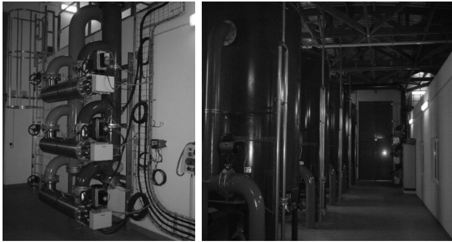
Figure 1.7. UV reactors and filters
