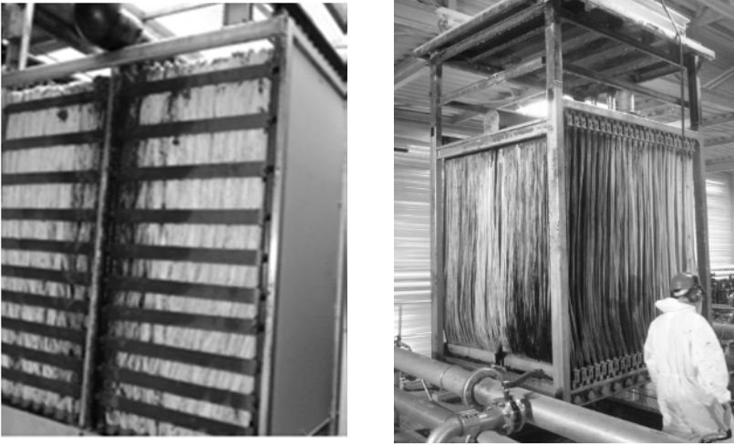
Figure 1.19. Clogging of immersed membranes
