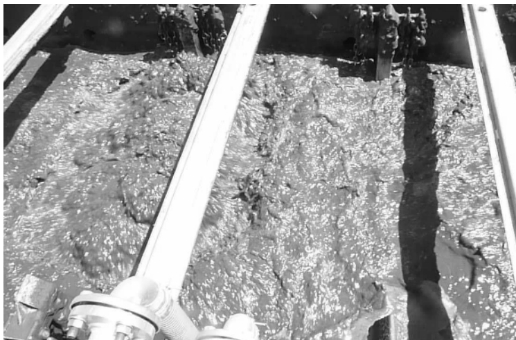
Figure 1.26. Non-aerated membrane tank
