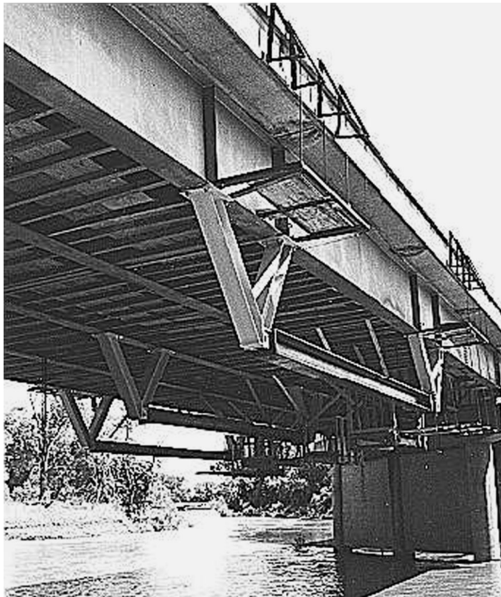
Figure 1.12 Highway I-35 bridge with semi-active dampers (Patten, 1998)
