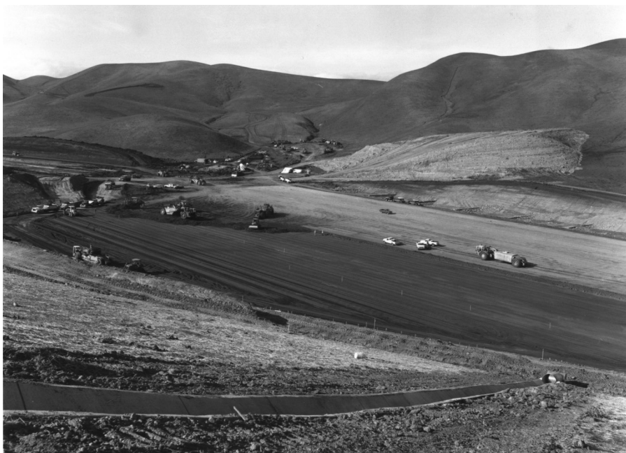
Figure 5-25 Development of large ravine landfill site. Equipment is compacting sub-base of landfill in preparation for placement of geomembrane liner.
