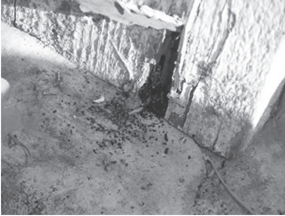
Figure 1.38 Drywood termites on a wood post base (© Specialty Termites, Inc.).
