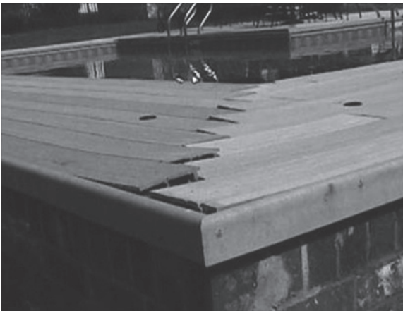
Figure 1.30 WPC deckboards distortions, swelling, and buckling.
