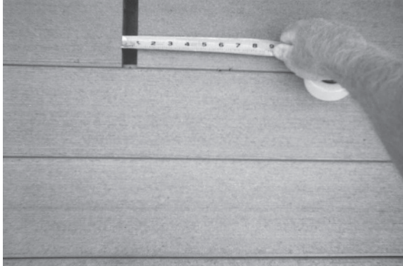
Figure 1.26 An 1-in. gap due to shrinkage of composite deck boards on a deck.
