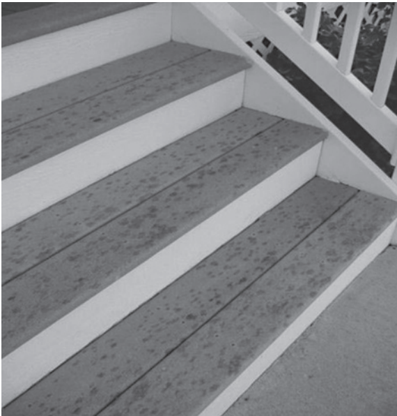
Figure 1.33 Mold stains on a WPC.
