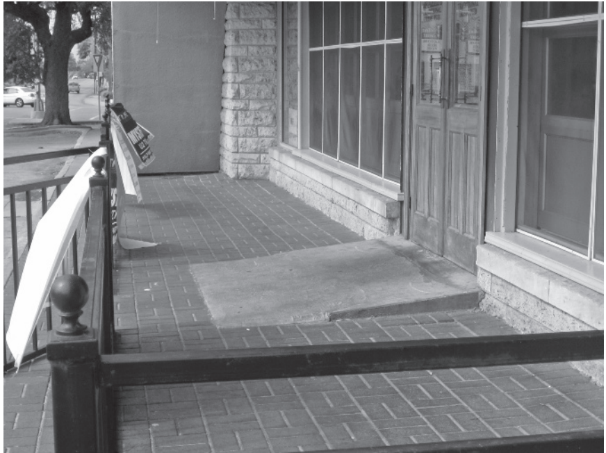
Figure 1.24: This exterior door does not have the proper slope at the landing and could benefit from a power-assisted door opener that will keep the door open if the power is off.
