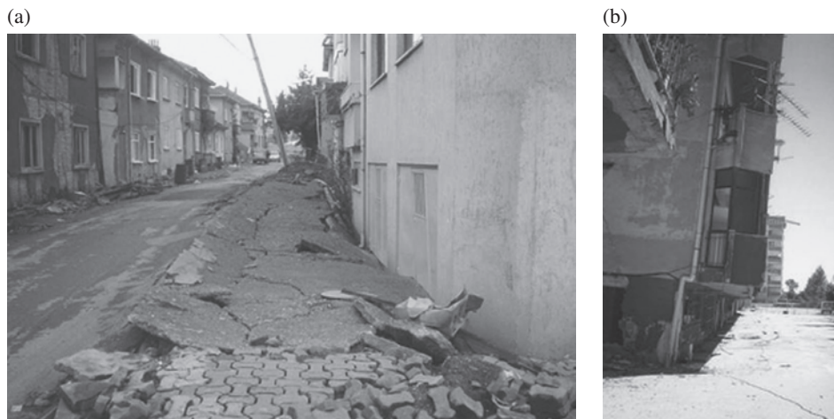
Figure 1.29 Damage observed during the 17 August 1999 Kocaeli in Adapazari (a) and Izmit in Turkey (b).
