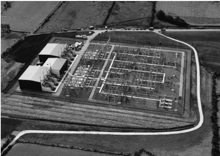
Figure 1.2 Terminal station of Moyle HVDC interconnector (Bipole 2 \times 250 MW, \pm 250 kV, with light triggered thyristors, commissioned in 2001). Reproduced with permission of Siemens.
